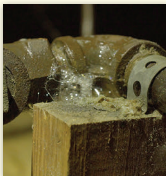
The leaking steel piping was tested, disconnected and replaced with TracPipe CounterStrike® all within 3 hours.
